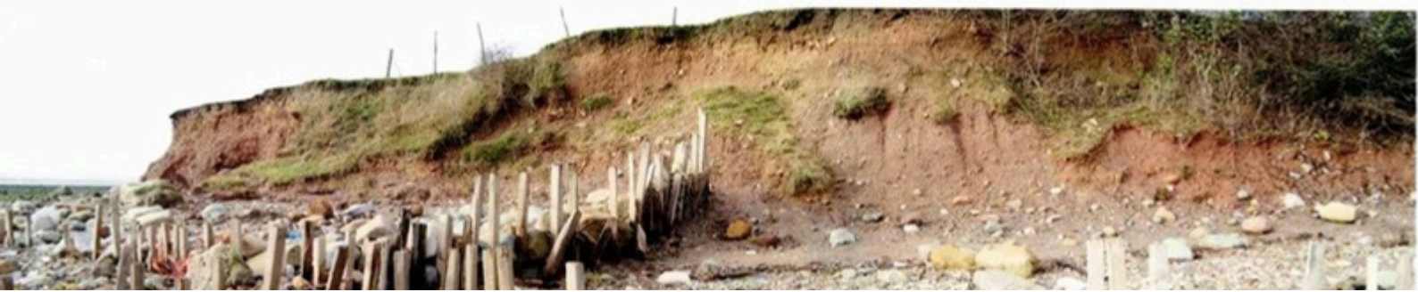
Erosion at Point End before the rock armour was installed.
